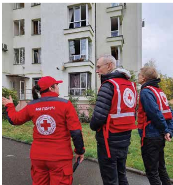
Canadian Red Cross Country Representative in Ukraine, Robert Laprade (centre), and Program Support Officer, Nikita Gorskyi (right), observe a damaged apartment building in Kaniv after an explosion with Yuliya Kholodna, the head of the Ukrainian Red Cross Society’s Cherkasy regional branch.
