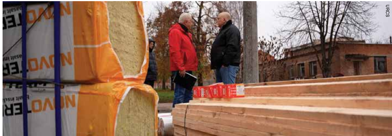
Donors to the Heal Health Centres initiative provided much-needed building supplies to help repair the roof of a maternity hospital in Sumy.
